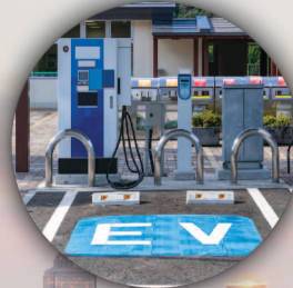
EV Charging Station
