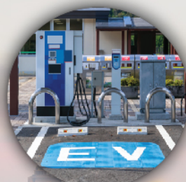
EV Charging Station
