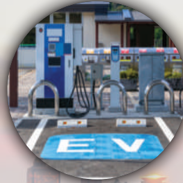
EV Charging Station
