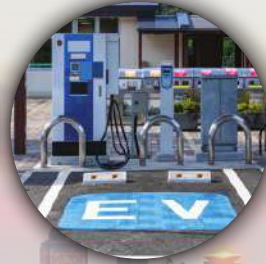
EV Charging Station
